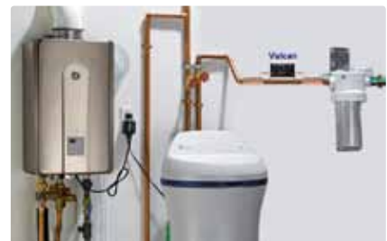
Vulcan installation with water softener
