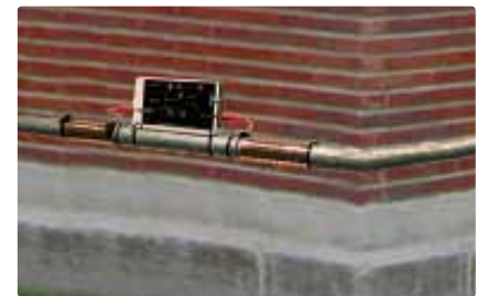
Vulcan outdoor installation
