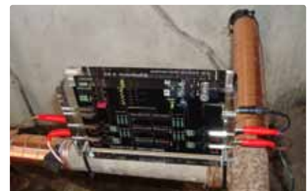
Vulcan installation in an apartment building
