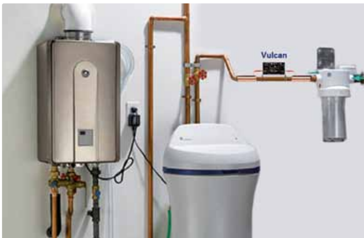
Vulcan installation with water softener
