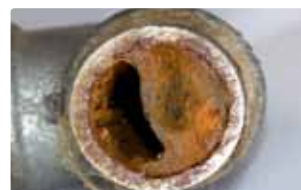
Pipe with scale deposits
