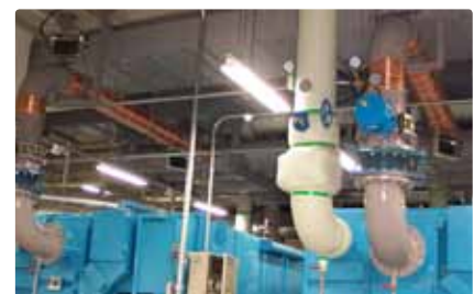
Vulcan installation in a factory
